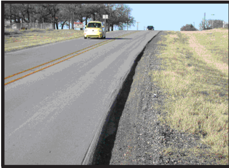
Figure 2. Maintenance personnel define edge drop-offs in risk-based terms with respect to two functional criteria: 1) the impact on safety of the traveling public, and 2) the potential for damage to the road.
