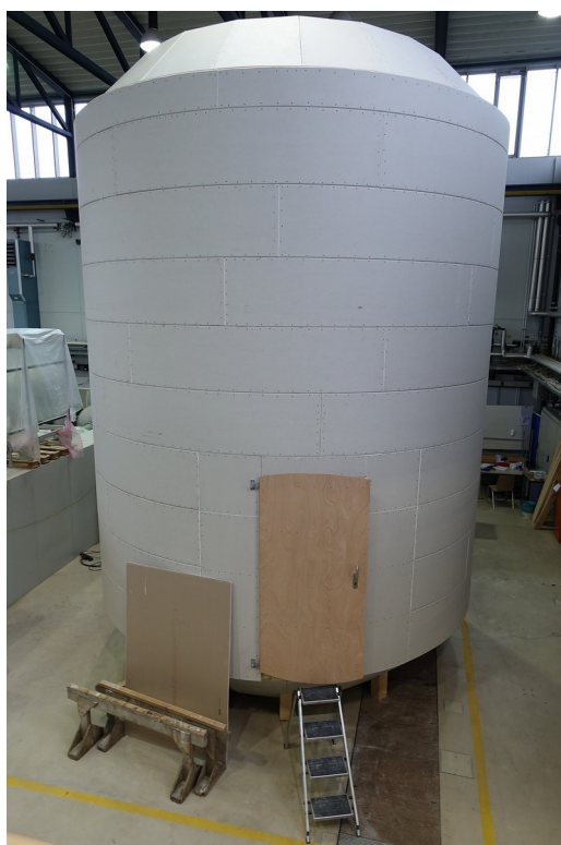
Figure 4. Mock-up version of the base module during construction. Approximate outer dimensions: height 6.5 m, diameter 5.2 m. The interior is split into 18 segments, such that the overall floor layout is almost circular, but the walls consist of plane, rather than curved panels. As shown with module 2 in Figure 1, the module has three doors (in the mock-up, one of the doors is blind), and the walls between the doors are lined with custom-made racks (see section VI). The longest continuous wall section houses 7 racks which carry biological and materials science equipment, and the second longest section houses 4 neighboring racks with the geological equipment. The shortest section is occupied by the stairs leading to the upper floor which serves no specific purpose during the test runs, but is intended for communication and a medical bay area later on. At the time of writing, the racks are being assembled – first photos of the equipped interior are expected to be available during the conference.
