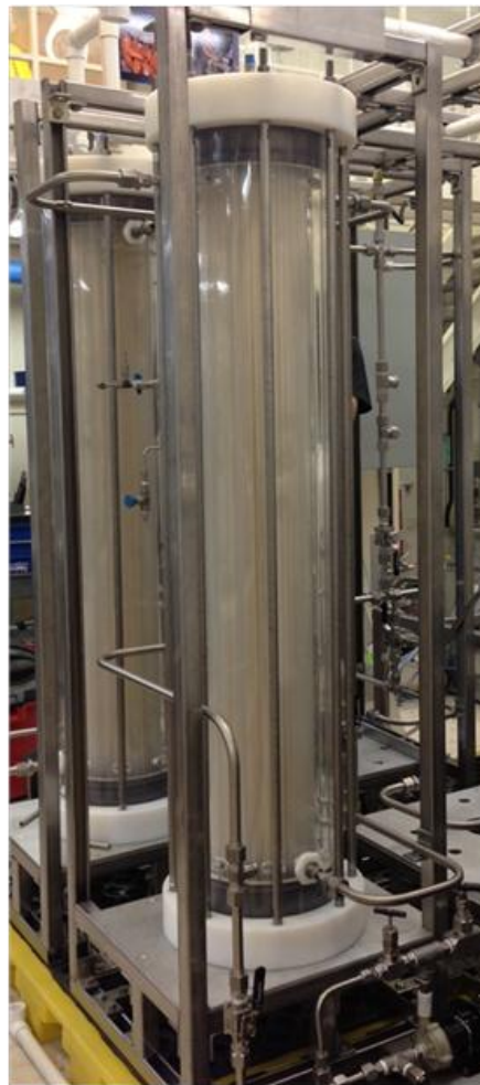
Figure 1. Assembled and installed MABR
