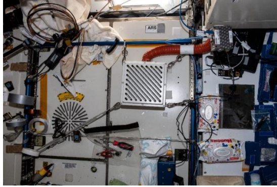
Figure 8. Brine Processor Assembly with BPA Exhaust Filter Attached.
