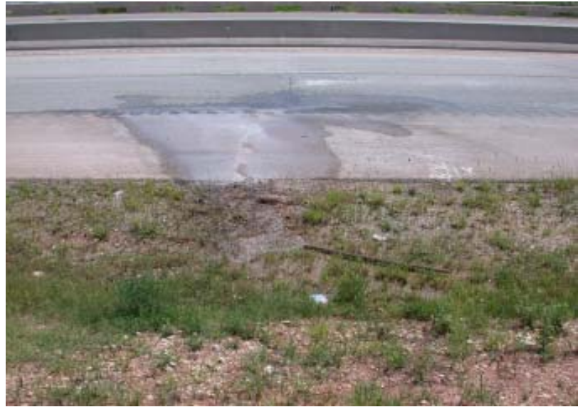
Figure 3. Water Seepage at the US-83 Overpass Bridge Departure Over Antilley Road in Abilene District.
